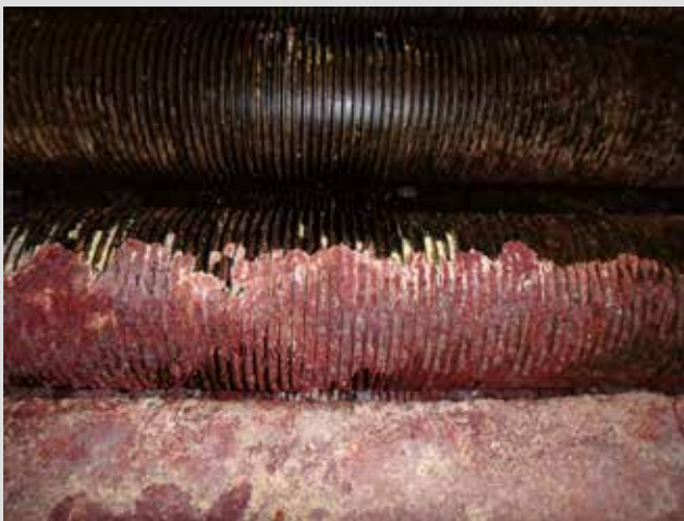
BEFORE - Heavy Fouling on a Convection Section
